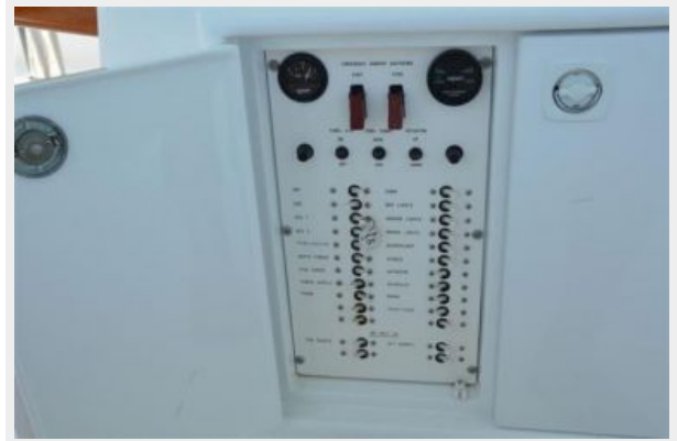
58 Davis Bridge Electrical Panel
