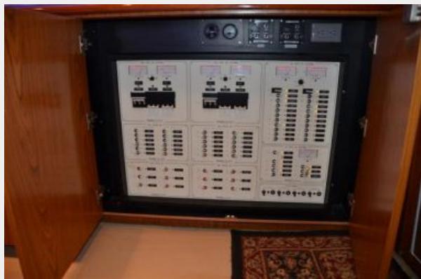
58 Davis Electrical Panel
