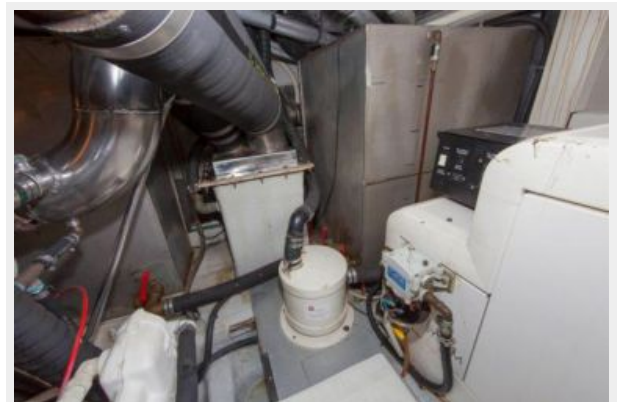
Engine Room Starboard Aft
