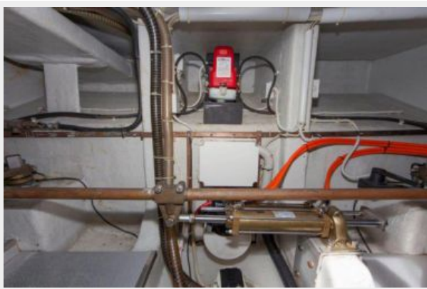
Lazarette Aft Bilge
