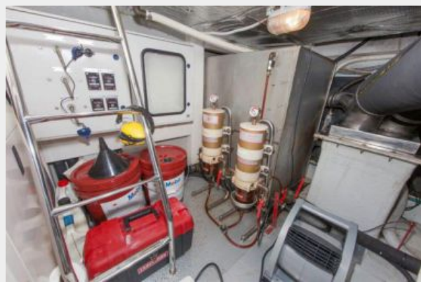
Engine Room Port
