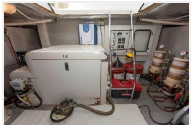
Engine Room Aft
