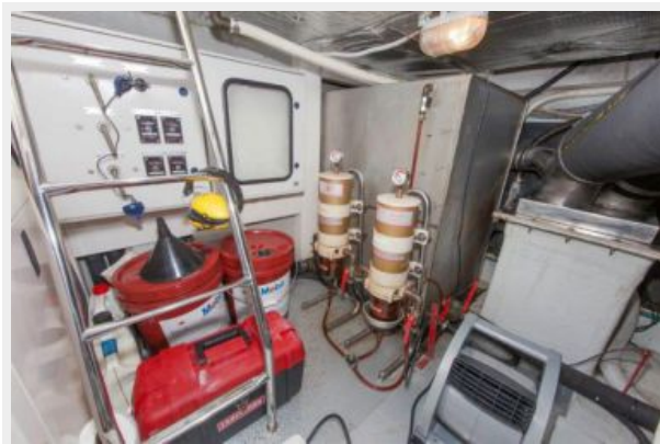
Engine Room Port
