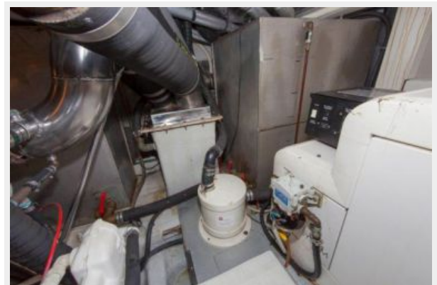
Engine Room Starboard Aft
