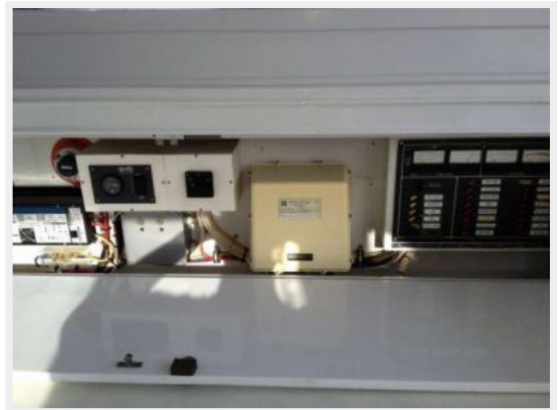
Starboard Breaker Panel
