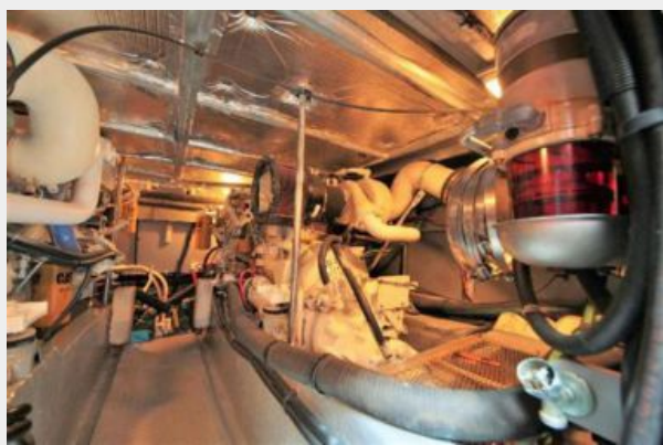
Sea Ray 480 Sedan Bridge Engine Room
