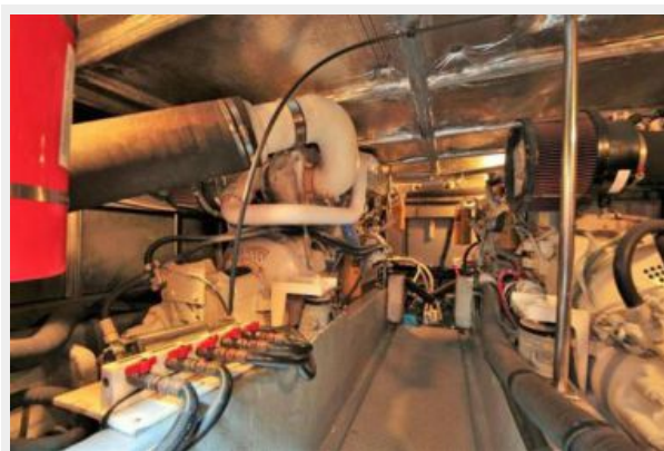
Sea Ray 480 Sedan Bridge Engine Room2
