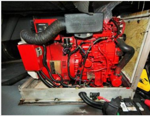
Sea Ray 480 Sedan Bridge Generator
