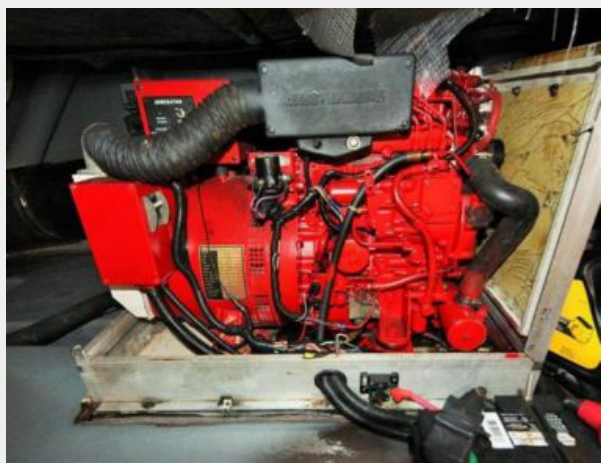
Sea Ray 480 Sedan Bridge Generator
