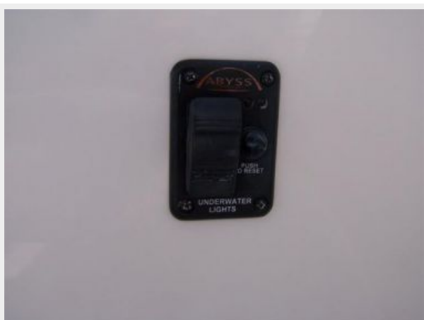
Underwater Lights Controls
