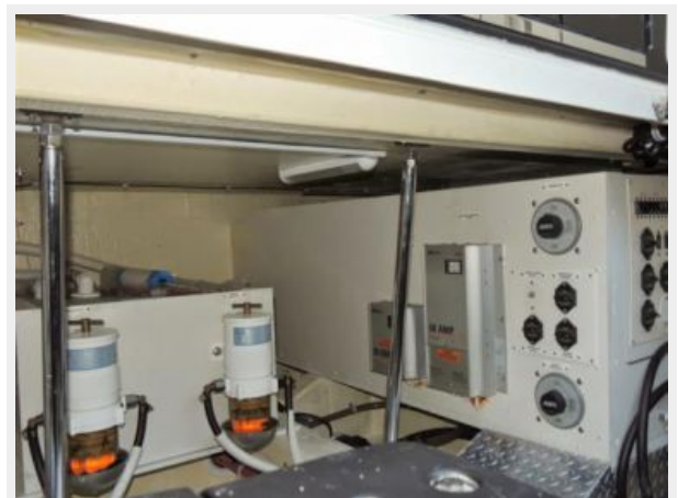
Starboard Engine Room Forward
