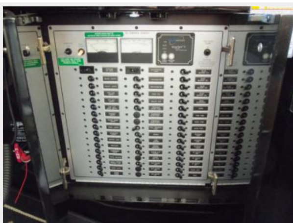
DC Electrical Panel at Helm
