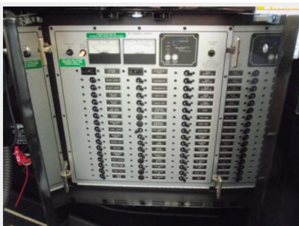
DC Electrical Panel at Helm
