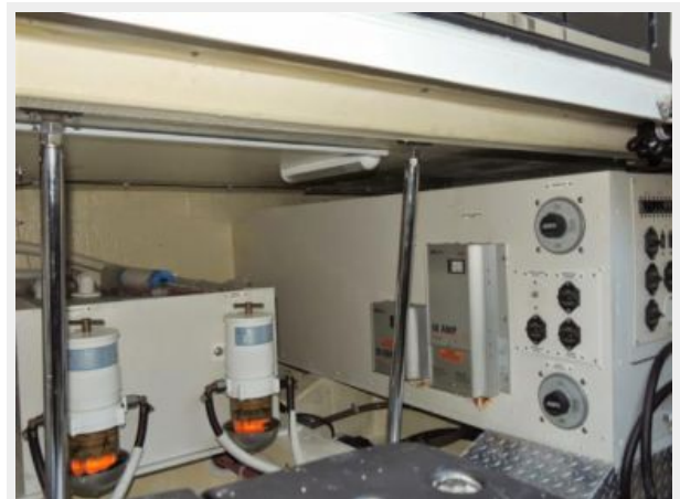
Starboard Engine Room Forward
