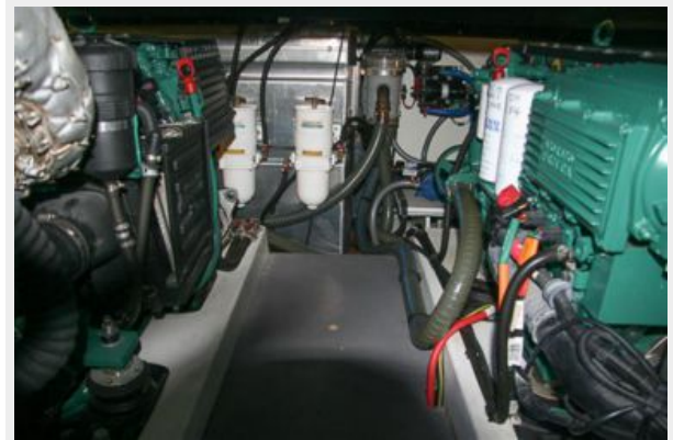
Clean Engine Room
