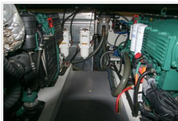
Clean Engine Room
