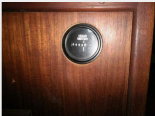
690 Hrs On Hobb Meter (installed 1999)
