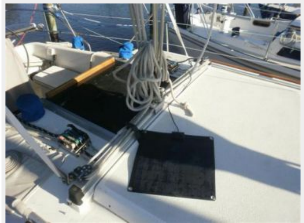
Small Solar Panel Keeps Batteries Topped off
