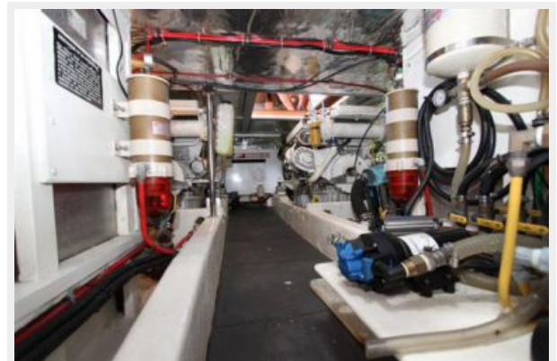
Engine Room Aft
