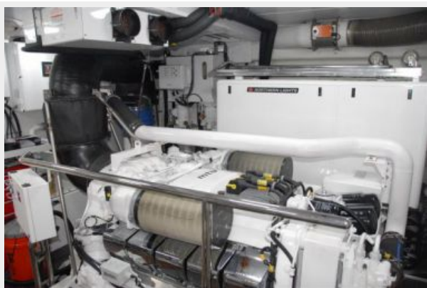
A/C Engine Room
