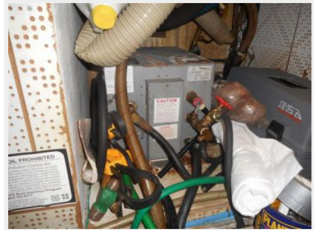
36' Marine Trader water heater
