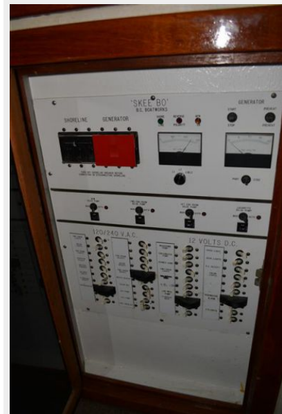
Fagley Electrical Custom panel
