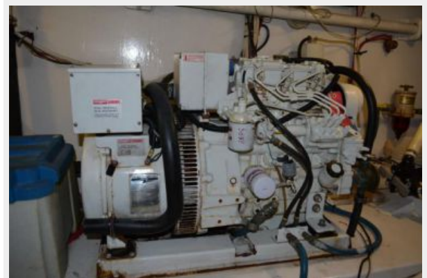
12 kw Northern lights generator
