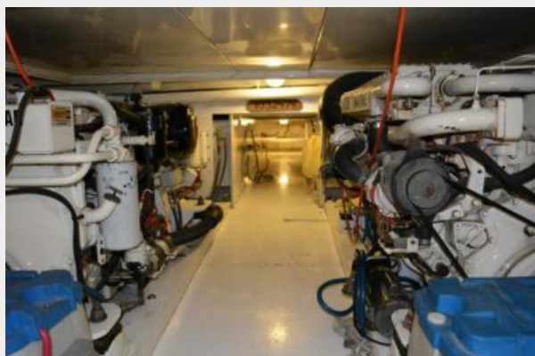
Easy access from generator to rudder shelf
