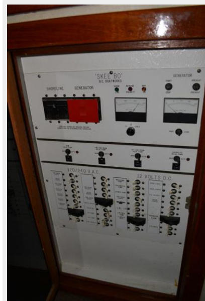
Fagley Electrical Custom panel
