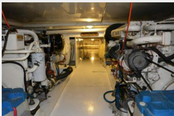
Easy access from generator to rudder shelf
