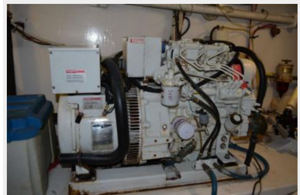
12 kw Northern lights generator
