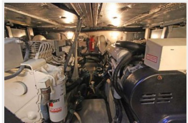
Engine Looking Aft
