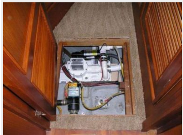
access to vacuflush system
