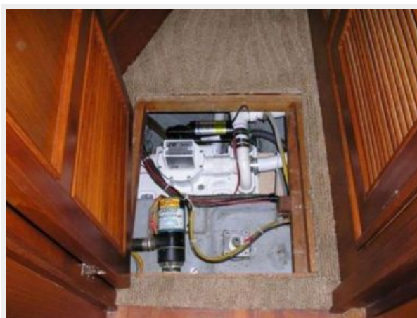
access to vacuflush system
