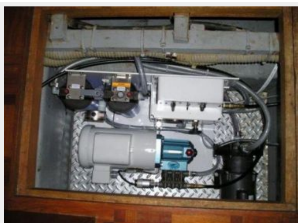
brand new water making system
