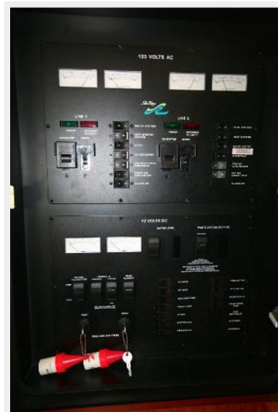
Breaker panel with ignition
