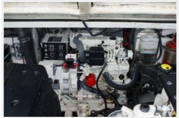
Westerbeke 5KW genset
