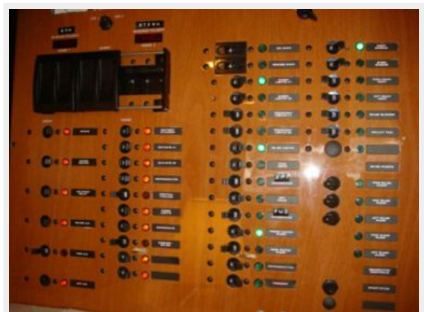
43' Mainship electrical panel1
