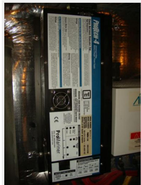
43' Mainship battery charger
