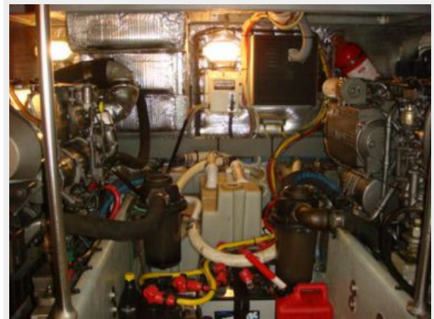
43' Mainship engine room
