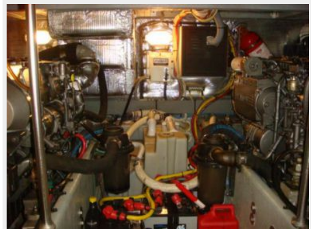
43' Mainship engine room
