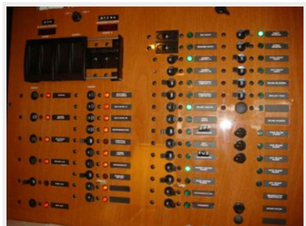
43' Mainship electrical panel1
