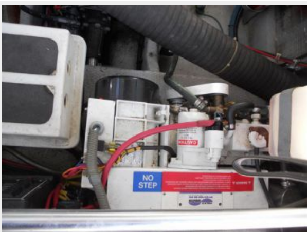
34' Mainship Pilot Express Engine Room
