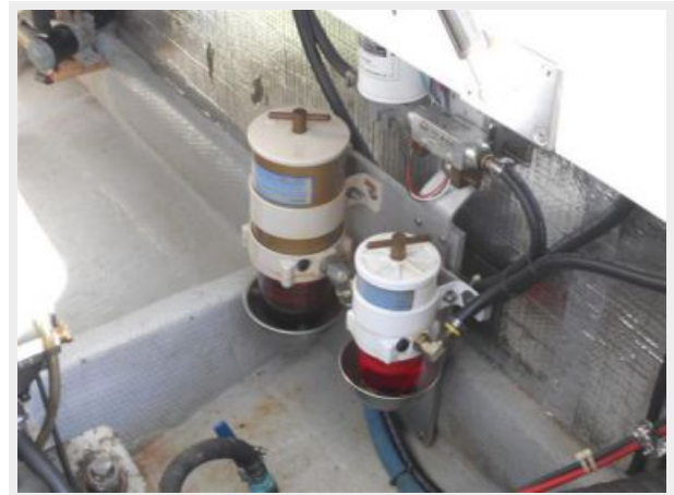
34' Mainship Pilot Express Engine Room
