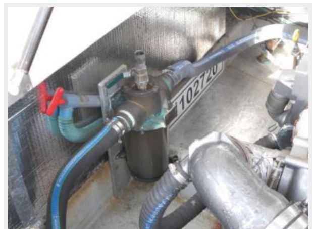
34' Mainship Pilot Express Engine Room
