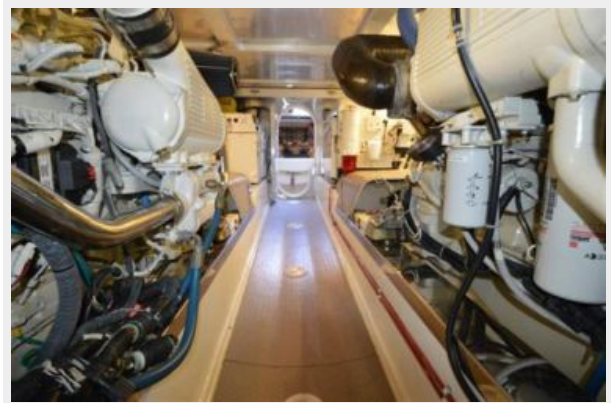
55 Fleming, Engine Room Looking Forward
