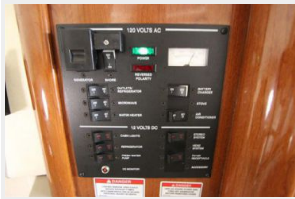
AC/DC Electrical Panel
