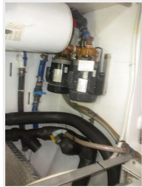
Dual A/C Sea Water Pumps
