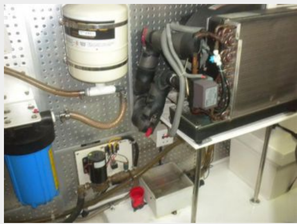
A/C Engine Room
