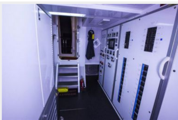
Generator Control Room
