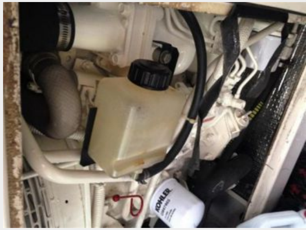
Kholer 12KW Generator
