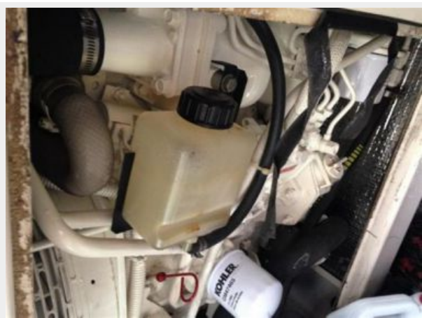
Kholer 12KW Generator
