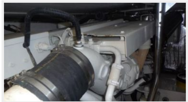
Engine & Mechanical Equipment 2
