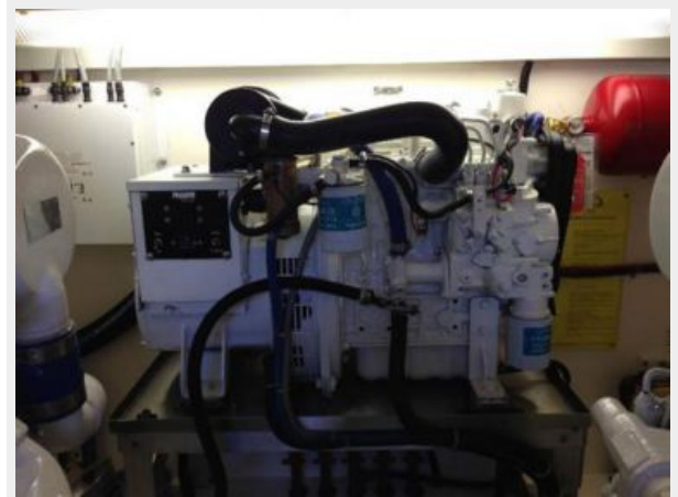
Auxiliary Generator Phasor
