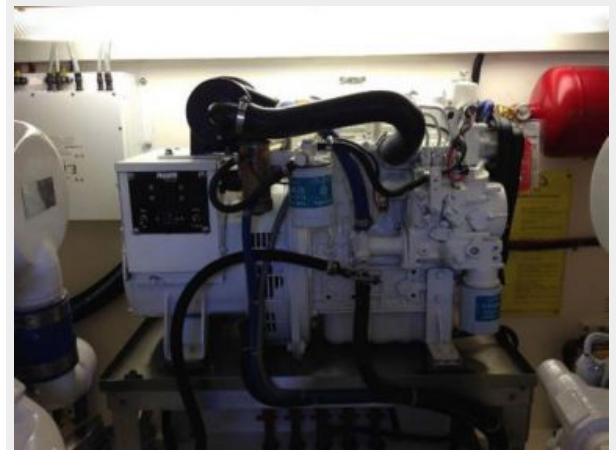
Auxiliary Generator Phasor
