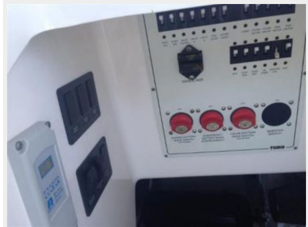
Engine Room Braker Panel
