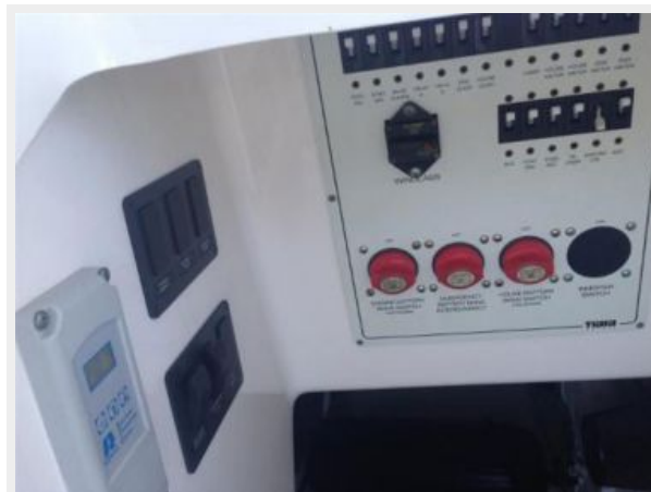
Engine Room Braker Panel
