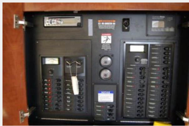
Electrical- Distribution Panel
