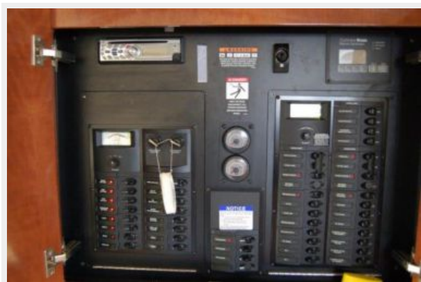
Electrical- Distribution Panel
