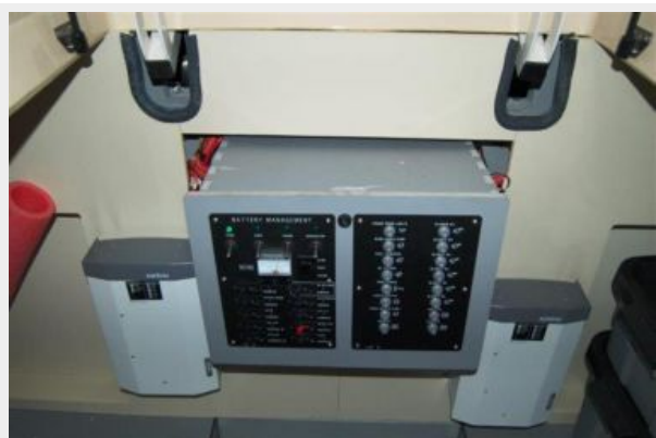
Electrical- Battery Mgmt System beneath Salon floor
