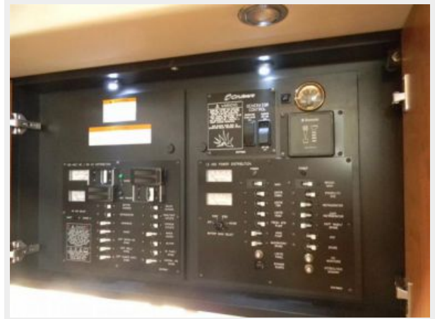
Main Distribution Panel
