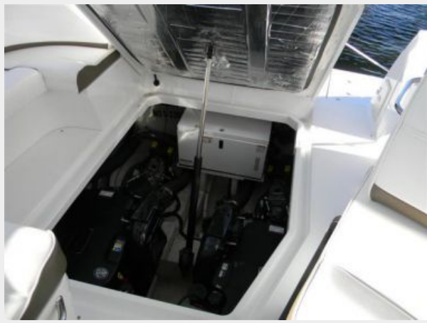
Engine Room Access
