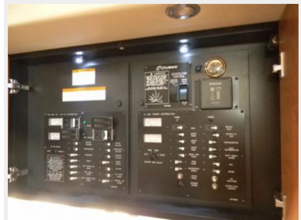
Main Distribution Panel
