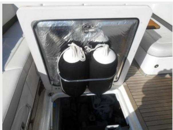
Engine Room Access
