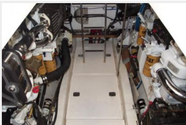
Clean Engine Room
