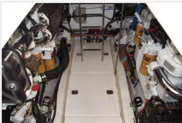
Clean Engine Room
