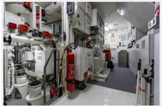
Engelberg Engine Room
