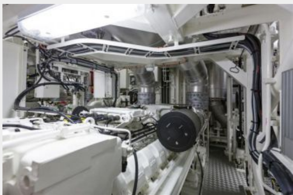
Engelberg Engine Room
