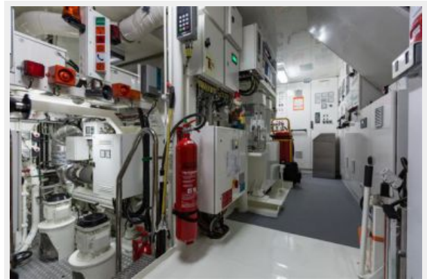
Engelberg Engine Room
