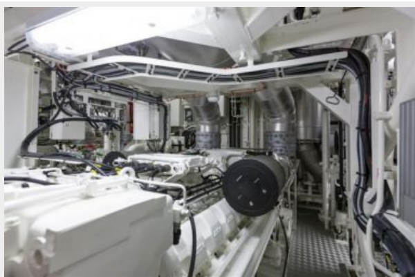
Engelberg Engine Room
