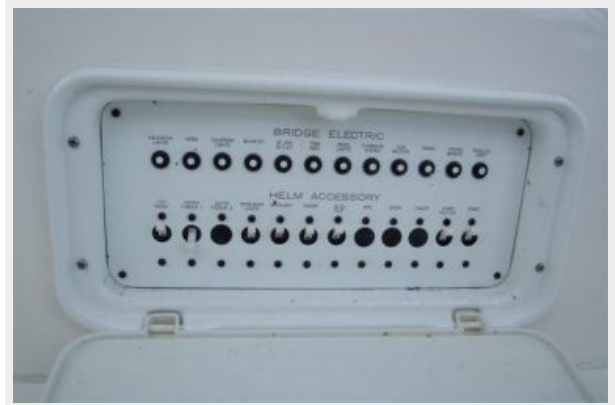
Flybridge Electrical Panel
